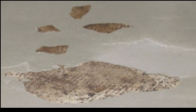
This is a photo of a leveling installation that went over existing mastic which was not properly removed...the mastic has profile...not just staining.
